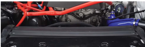
27. Remove the bolts that secure the AC condenser. Then, slide the condenser upward to free it from the tabs at the top. Lower the unit to give yourself some space to reach the intercooler. (2x 10mm bolts)
